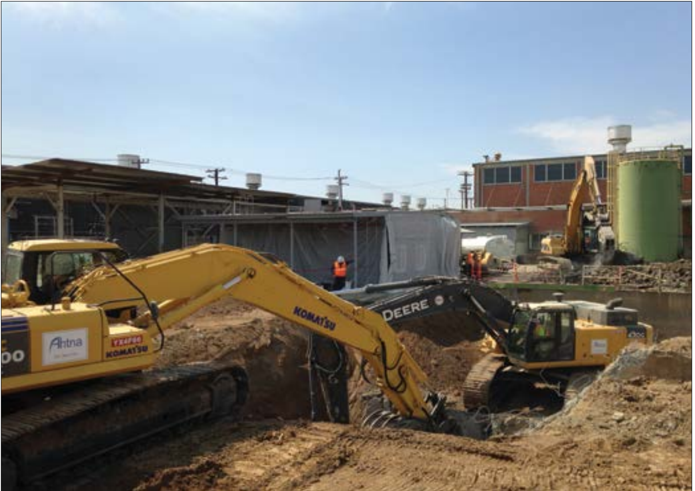
Excavation of the sand filter sump at the Riverbank Army Ammunition Plant, Calif. The facility was opened in 1942 and initially served as an aluminum reduction plant to support World War II aircraft manufacturing. PHOTOS COURTESY AHTNA ENGINEERING SERVICES
