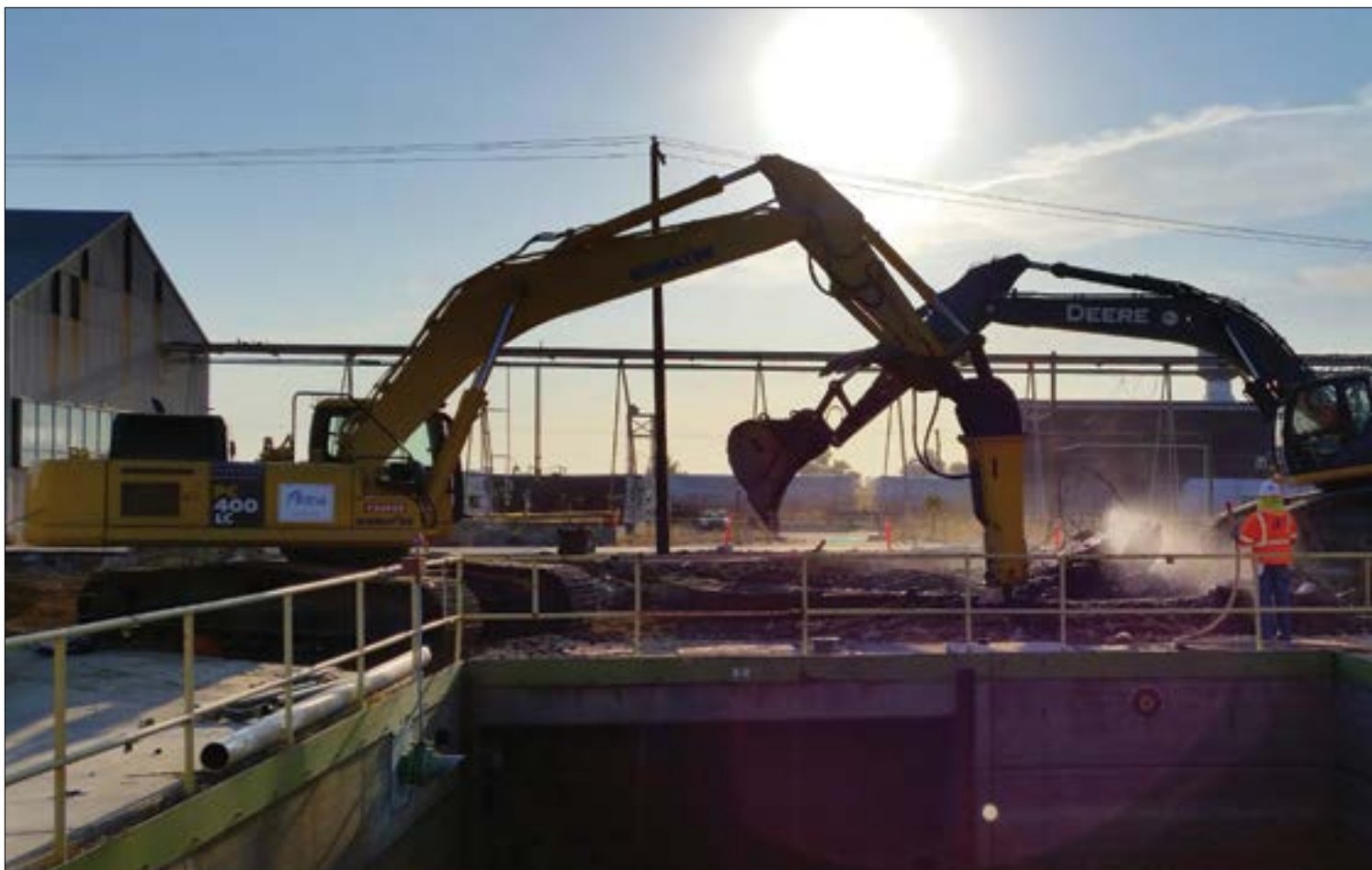
During Riverbank's long history, many upgrades were made, which created a complex infrastructure that combined both old and new systems. The site was put on the National Priorities List in 1990.
